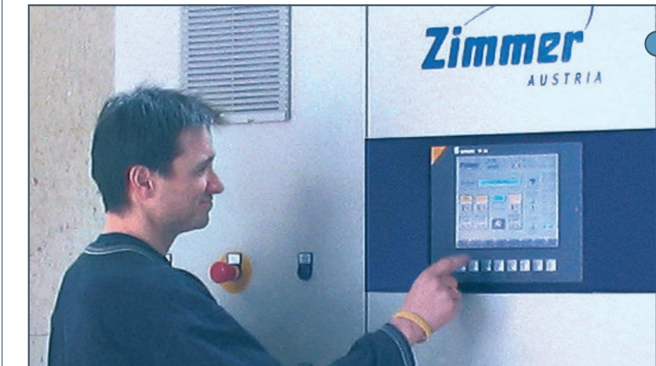
Central automation PLC-unit
